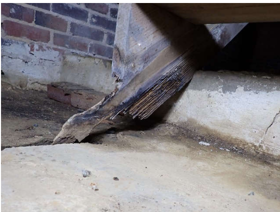
Picture 17 Basement stair stringer, rotted
