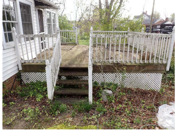
Picture 8 Side and front decks, poor condition
