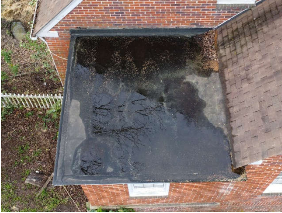
Picture 7 Standing water on flat roof, left rear addition
