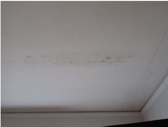
Picture 11 Water & cracking damage to interior ceiling
