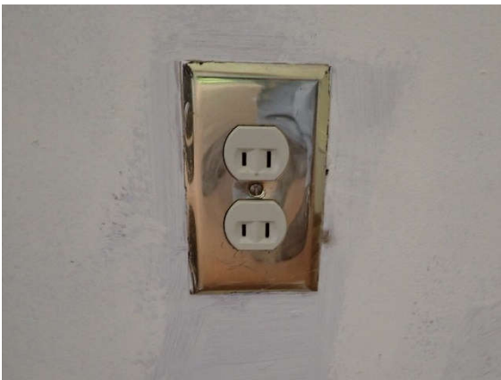
Picture 15 Non-grounded two wire receptacle (typical)
