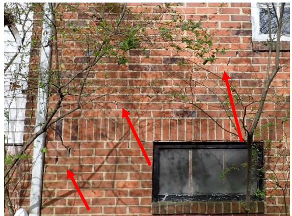
Picture 10 Veneer cracking, rear of house by corner
