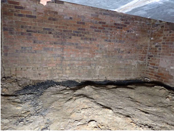
Picture 19 Moisture intrusion through front basement wall (typical)
