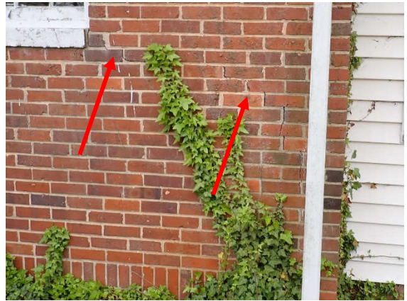
Picture 2 Veneer cracking at front of house, right
