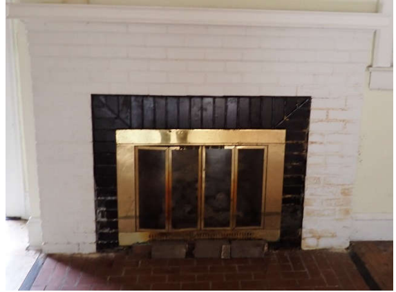
Picture 14 Moisture intrusion through fireplace brick (from exterior)
