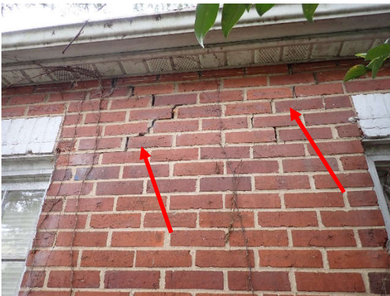
Picture 3 Veneer cracking at front of house, left
