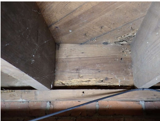
Picture 21 Termite damage, left side basement wall
