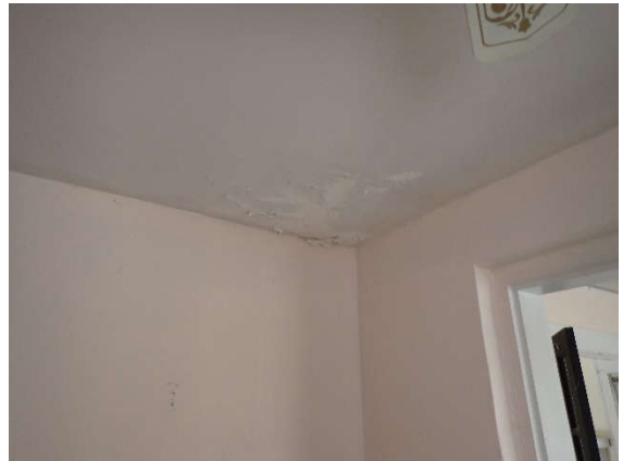
Picture 12 Water damage to interior ceiling
